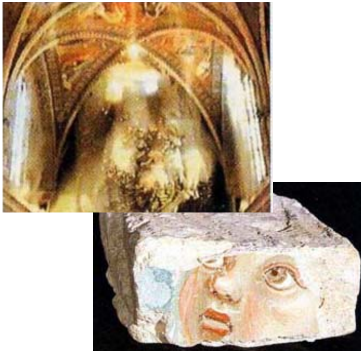
Collapse of S. Francesco d'Assisi vault – Assisi (PG)
